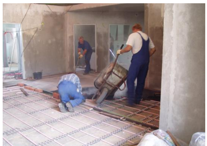
Camp site sanitary building Gross Quassow, 2005, installed by company Reinhard Schneider from Neubrandenburg, Germany
